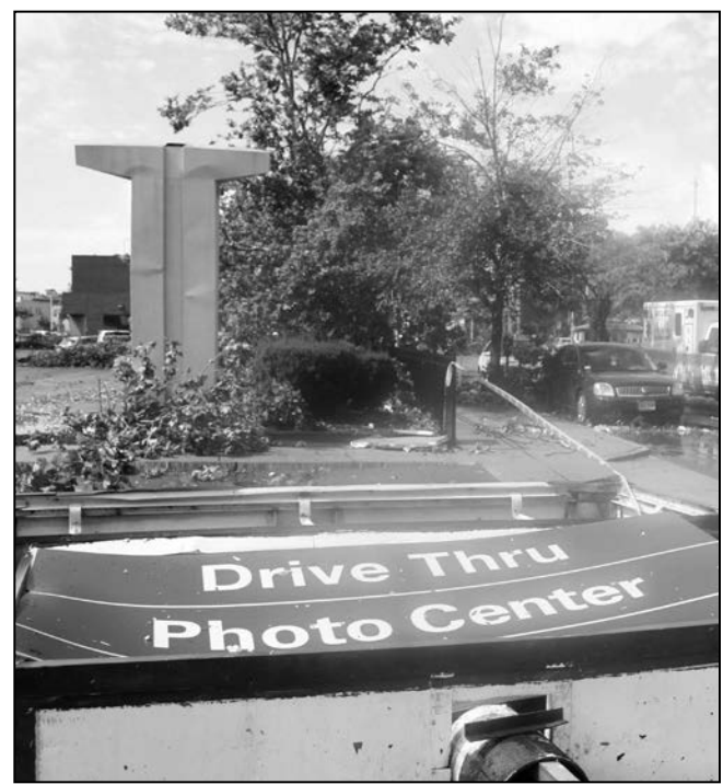
The Rite Aid sign on Broadway was ripped down with only part of it in the parking lot. Cars were stalling all over Broadway too as they had been inundated with water and debris.
