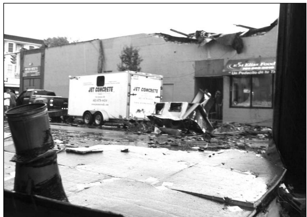
The roof from Peter Woo's Restaurant and the adjoining convenience store was transported across Park Avenue, leaving debris everywhere.
