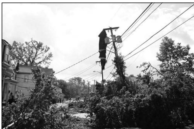
Trees made Mountain Avenue impassable and a piece of roofing material hung perilously from a pole with three electrical transformers.
