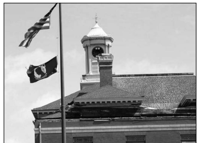
The American flag at City Hall hangs on by a thread as windows, the clock and the roof show the tremendous damage done to the Hall by the tornado. City Hall will remain closed until further notice.
